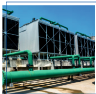
Compressors and Cooling Towers
