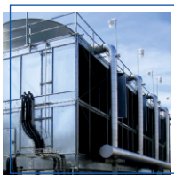
Cooling Towers & Chillers
