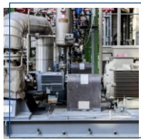
Hydraulics and Pumps
