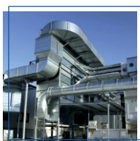
Pumps and Fans
