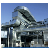
Fans & HVAC Systems
