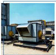
Fans & HVAC Systems
