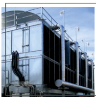
Cooling Towers & Chillers
