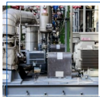
Hydraulics and Pumps
