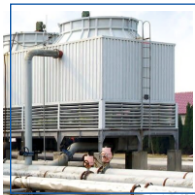
Compressors and Cooling Towers
